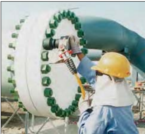
◀ Easy and reliable service in the field using Enerpac SQD-series torque wrenches.
